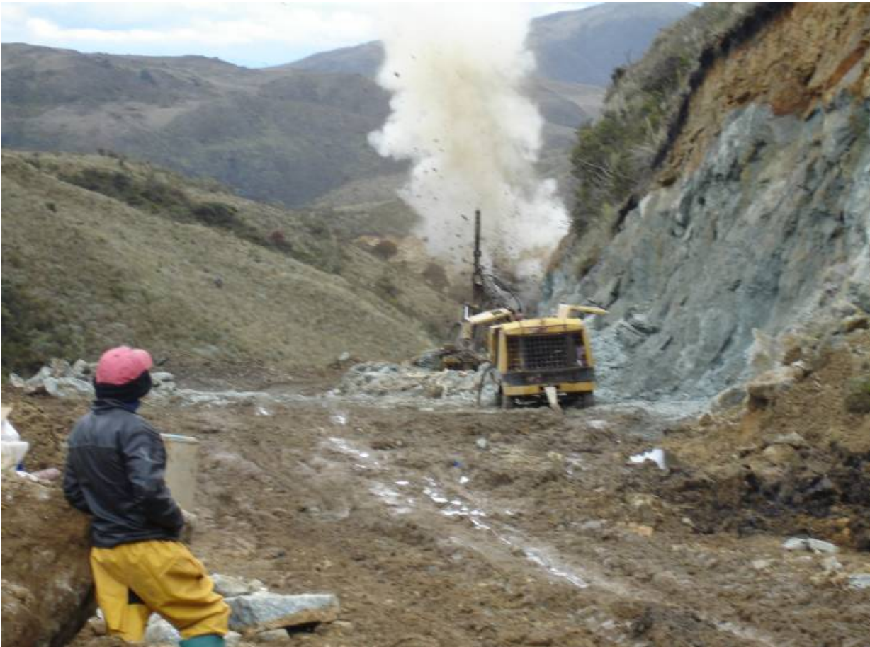
"Tirar piedras" (Falling rocks) at the Sigsig-Matanga road
